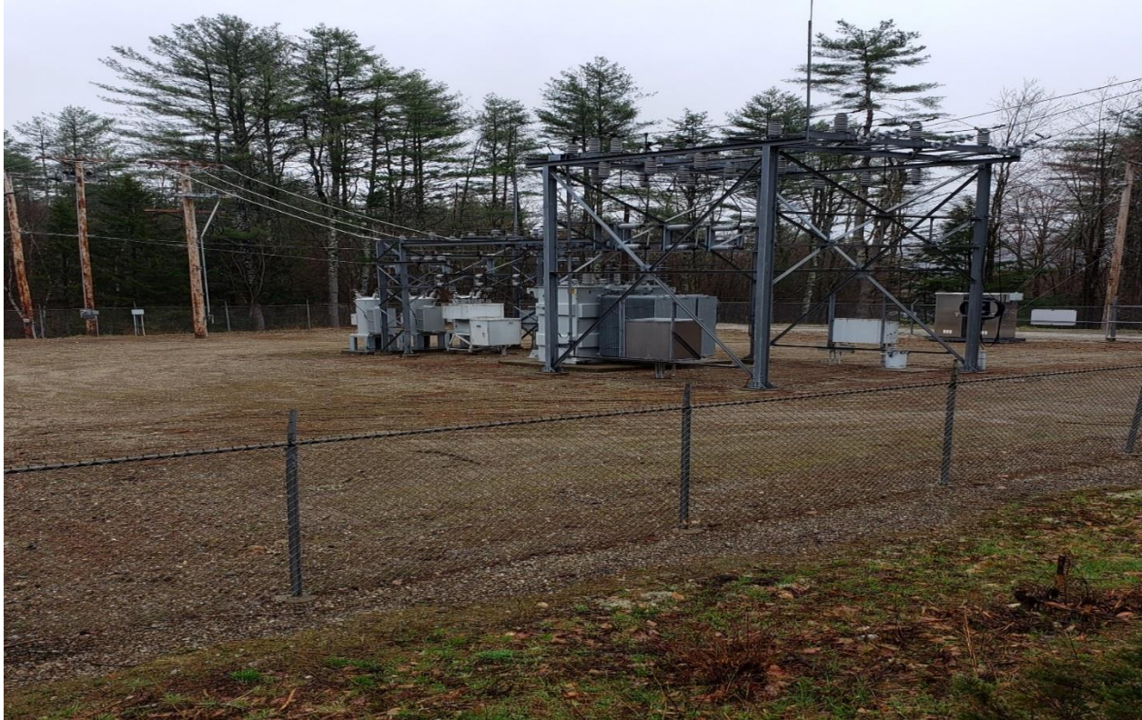
Figure 14 Ludlow's Smithville Substation
