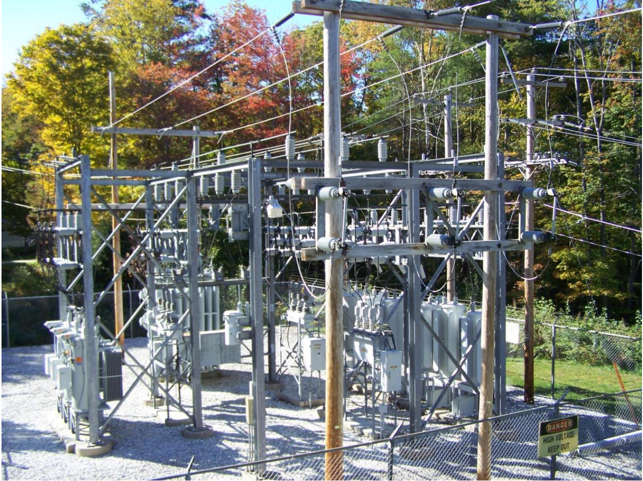
Figure 12 Ludlow's Route 103 Substation
