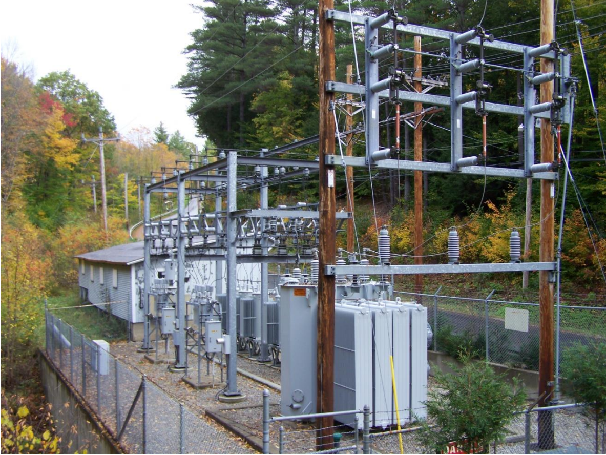
Figure 13 Ludlow's Commonwealth Substation
