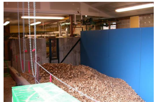
Figure 27: Wood chip heating system at Weathersfield School.
